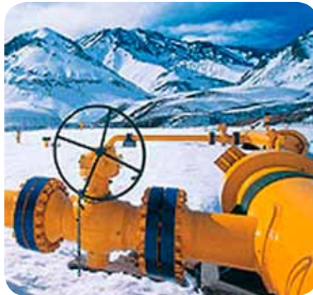
Fig. 5.3: A gas pipeline in Tierra del Fuego, South America. The world's most southerly natural gas production facility was put into operation in June, 2005 by the ownership consortium (Photo: BASF)
